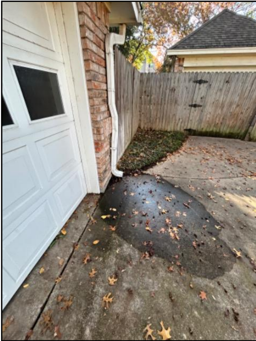
17. Discharge too close to building
