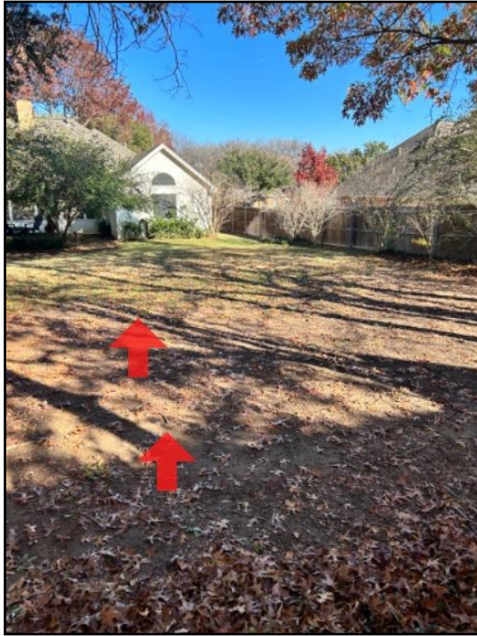
28. Water Drains towards the home
