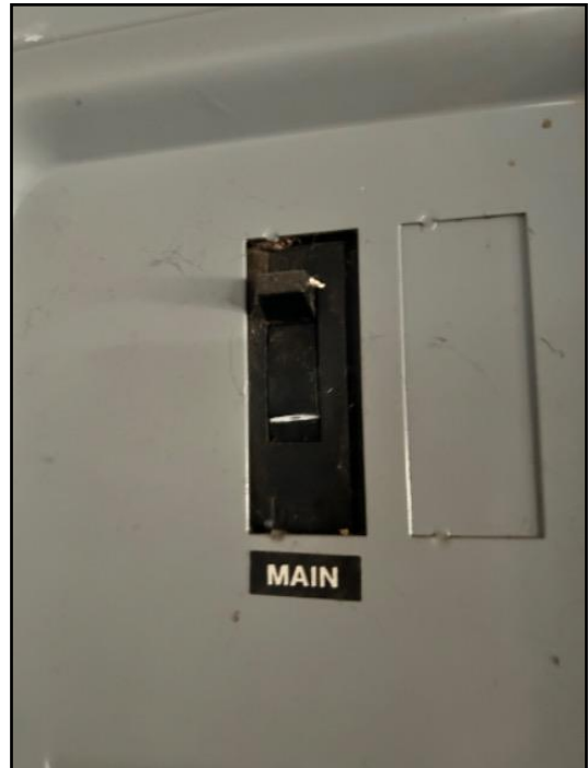
38. Main Shut Off
